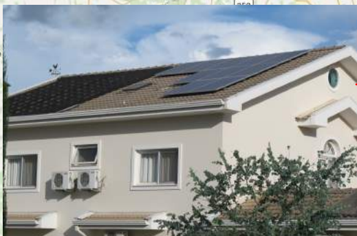
HOUSE OWNER UFV: 2.7 kWp – Mar/2015
